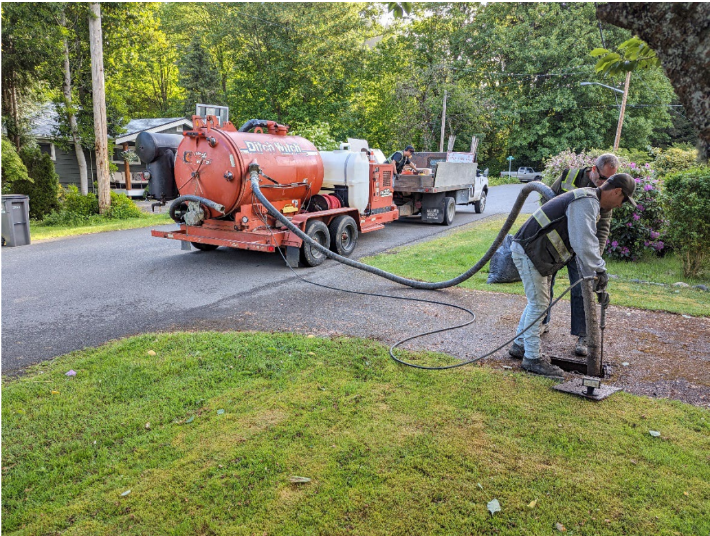
“Potholing” was undertaken within the water service box to determine the pipe material
